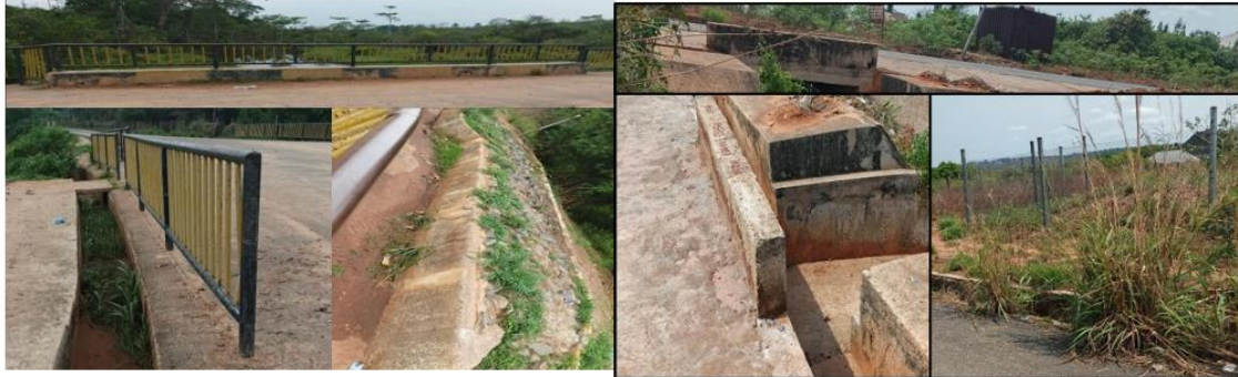
Fig x: A protective measures at Umuogele-Umuakwu and Amuda-Achara-Isuochi gully site
