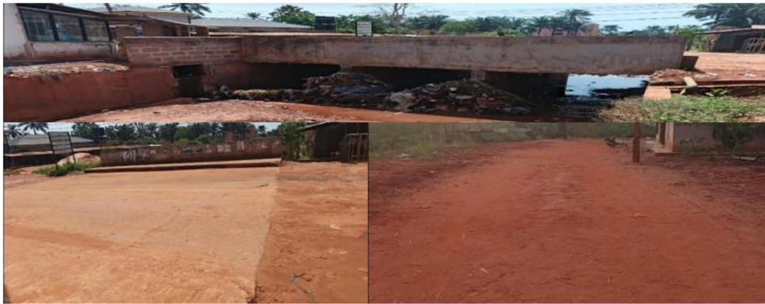
Fig viii: The Onuiyi erosion re-constructed bridge and recued roads at Ibeziako Street Onuiyi
