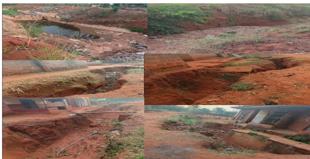
Fig xii: A view of emerging erosion gully at Onuiyi-Alor-Uno Nsukka gully erosion site Source: Field study (2025)
