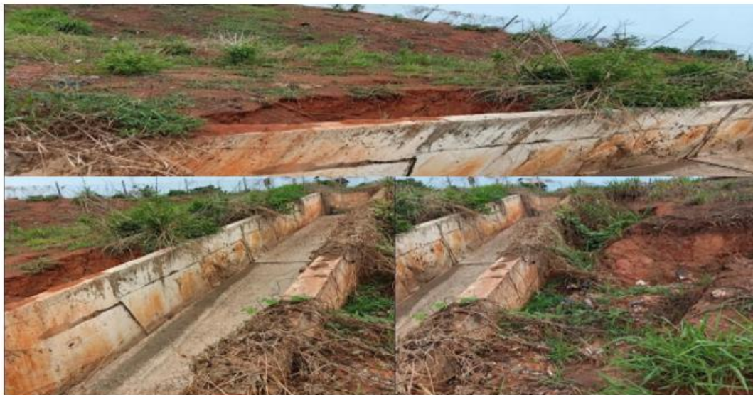
Fig v: Effects of scanty afforestation at Amuzukwu-Umuagu gully erosion control project
