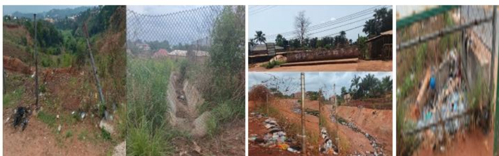
Fig ix: A view of the installed steel fence at Amuzukwu-Umuagu gully erosion sites
