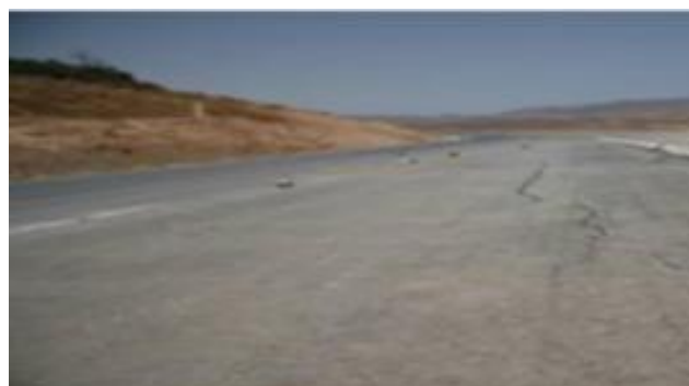
Fig 1: Cracks on the body of the roadway
