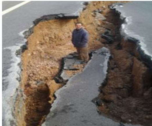
Fig 5: Deformation of the pavement body, PK 52+040~093
